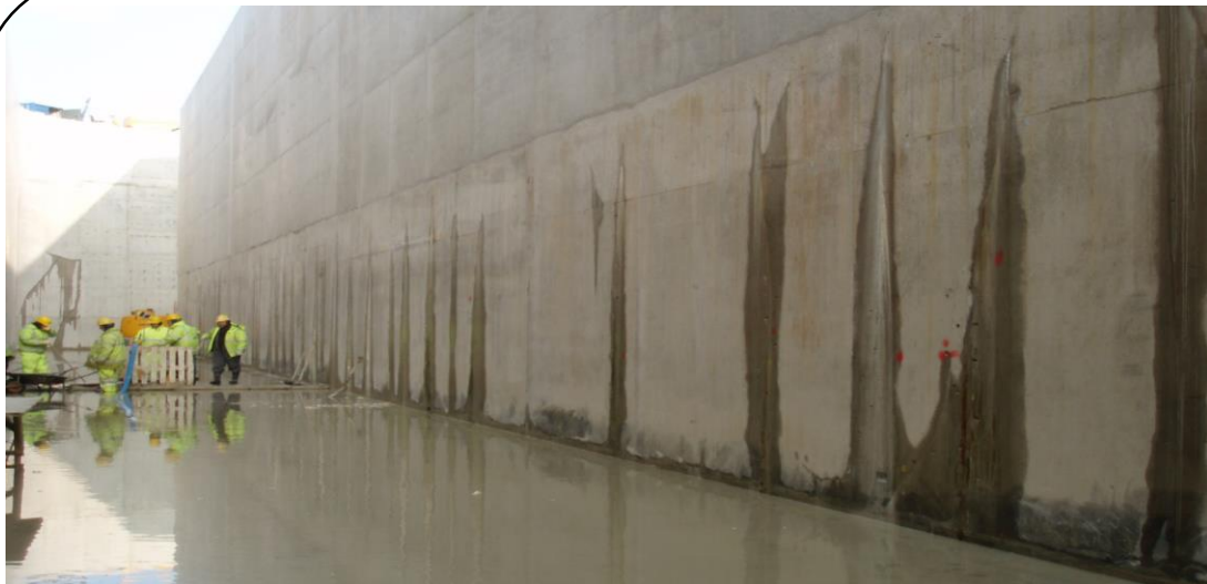
Example of Thermal Cracks in a RC wall
